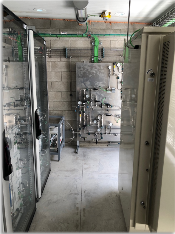
Roof top H 2 production plant
