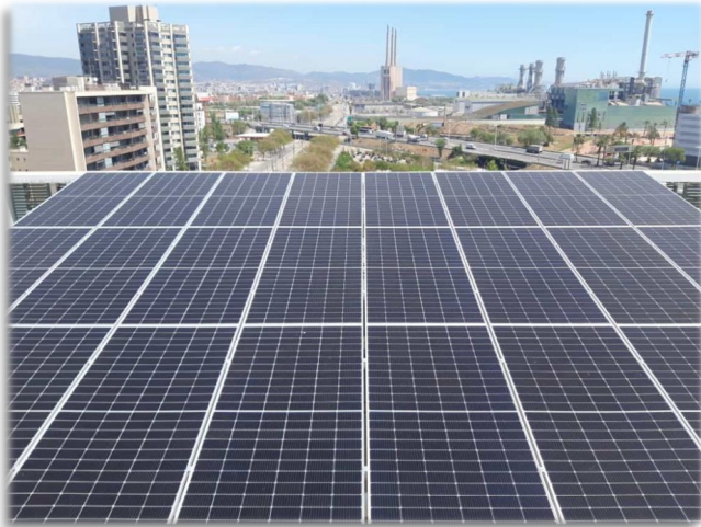
Solar Photovoltaic Structure
